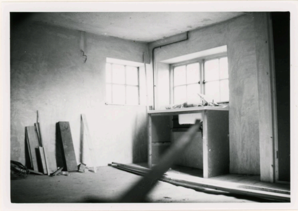
Kitchen, S.E. corner (see pic. on right). South window enlarged, sink moved to S. wall
