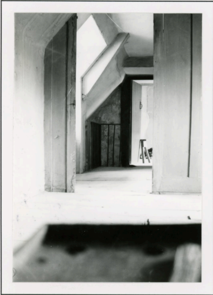
Main bedroom looking west to stairtop and second bedroom, through the door to matchboard partition which divided the main bedroom into two. Note flimsy banisters, rain streaks on walls. (1963).
