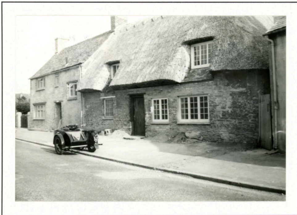
Altered: R.H. door becomes a window. R.H. window restored to original size. Thatch cut back upwards and renewed. (1963).
