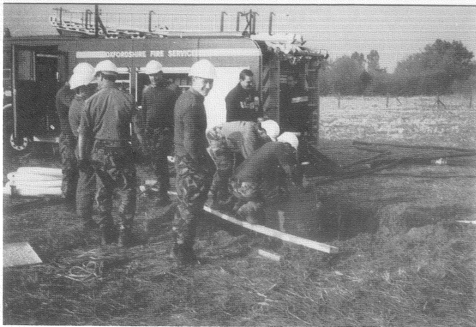
Bampton Fire Brigade help members of 218 Field Squadron with their task of installing the infrastructure needed for further development on the Buckland Road site.
