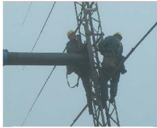
This picture gives some idea of the size of the centre support when it was lowered for maintenance
