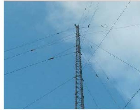
One end of a Triple Curtain Rhombic mast mounted. The triple connection is visible to the right of this mast
