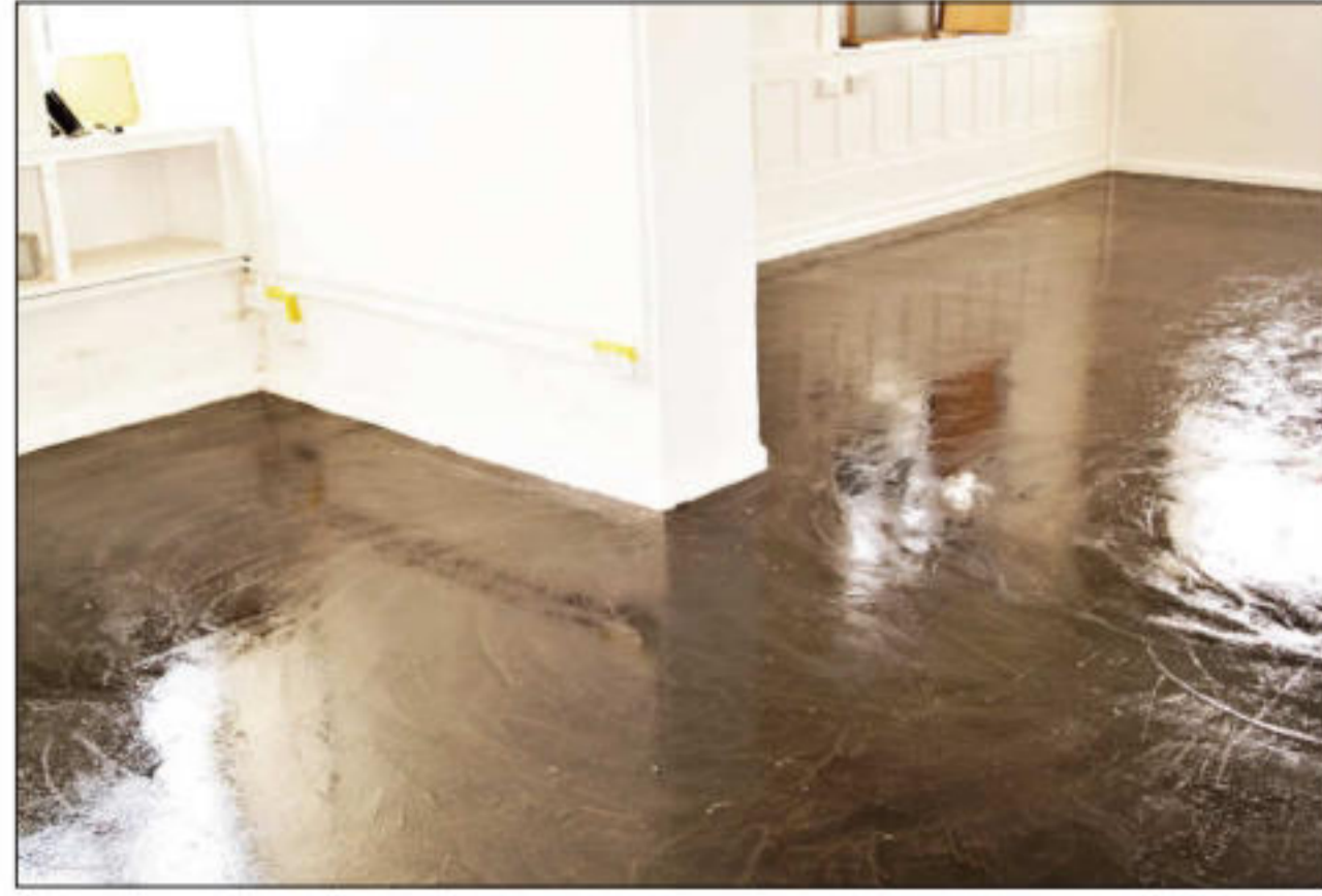
Damp proof to library floor
